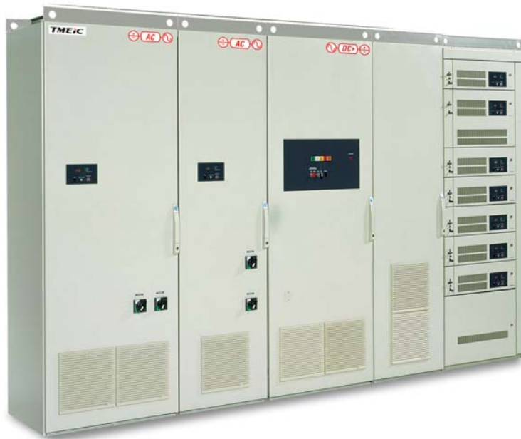
TMdrive-10 Variable Frequency Drives Cabinet
