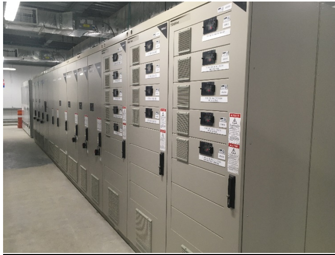
Drive system delivered by TMEiC
