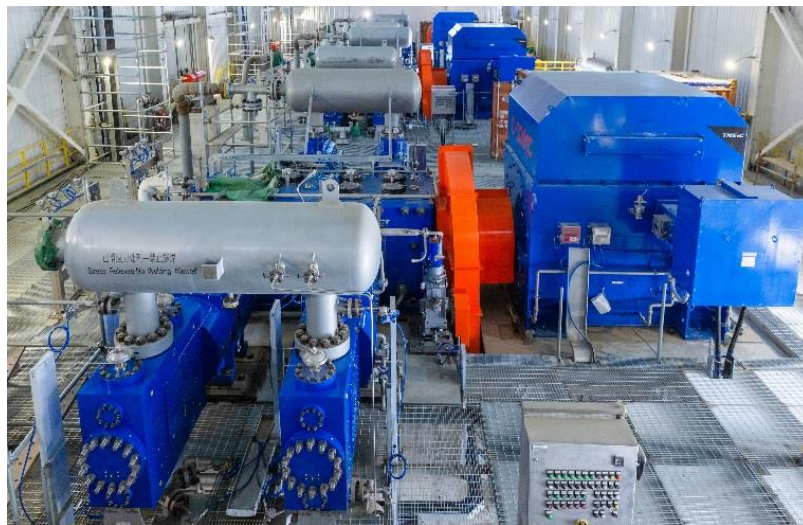
Reciprocating Compressor (left) and TMEIC Synchronous Motor (right)
