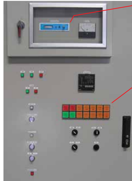
Interface and Water Cooling Panel
