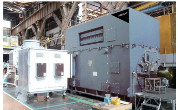
2-Pole Synchronous Generator 2P-88MVA, 13.8kV 60Hz | Pulp & Paper Plant
