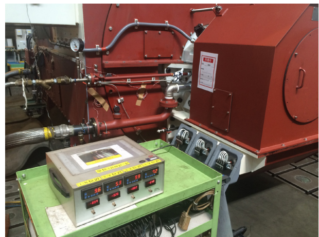
Figure 5. MV motor vibration test using proximity probes.
