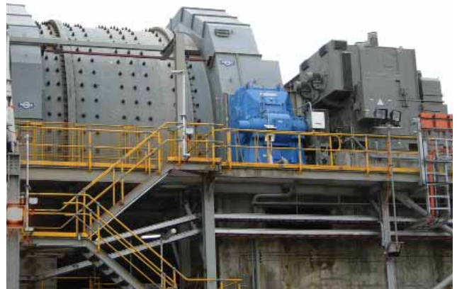
SAG Mill and Motor
