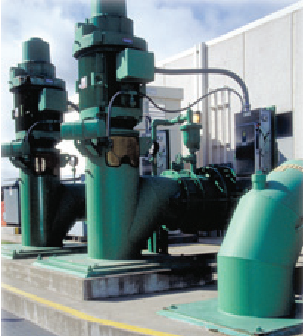
Typical vertical water pumps
