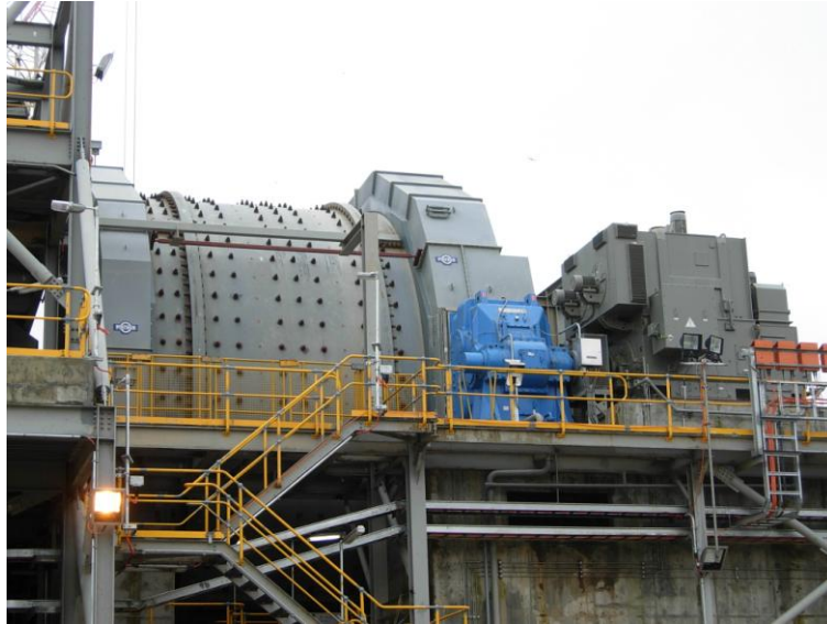
Wound Rotor Induction Motor driving a Grinding Mill
