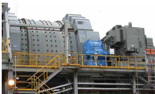
SAG Mill and Motor
