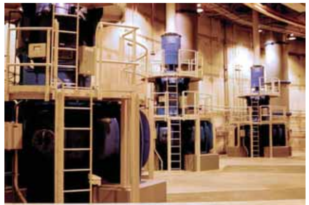
Large pumps in a Water Treatment Plant
