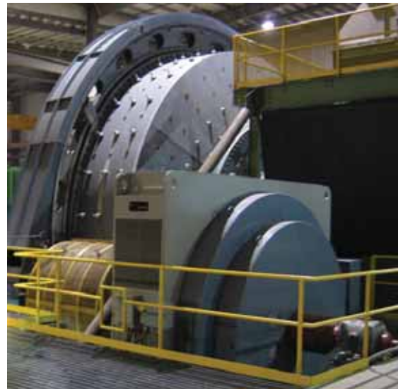
SAG Mill and Motor
