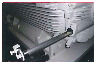
Waste Grease Removal System
