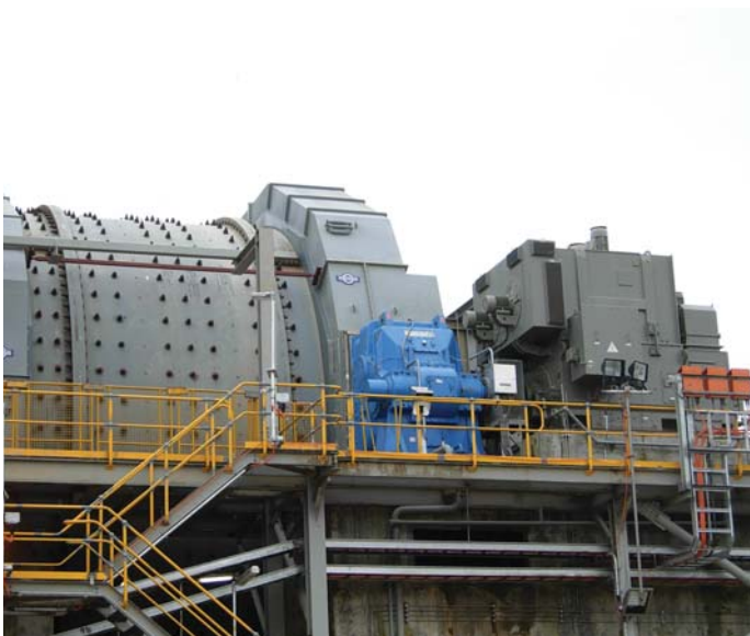
Wound Rotor Induction Motor Driving a Grinding Mill
