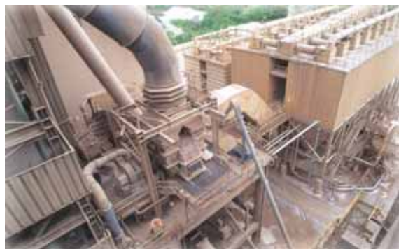
Induced Draft (ID) Fan
